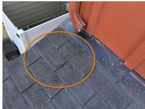
Heavy granule loose under downspout
