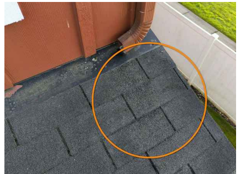
Heavy granule loss under downspout
