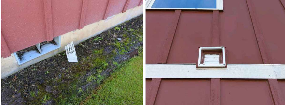
Here's the screen laying on the ground that fell off of the dryer vent termination Dryer vent on right side of home
