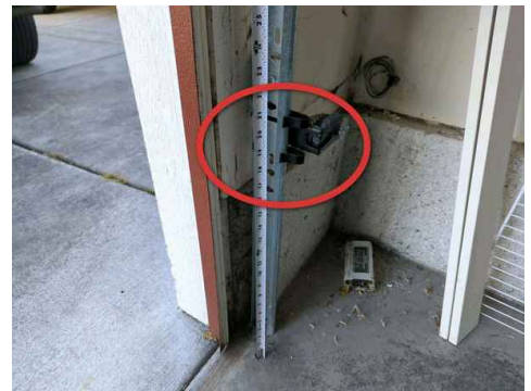
Photo sensors installed too high
