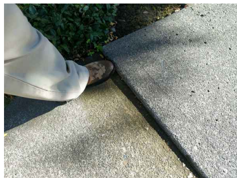
Offset is a trip hazard
