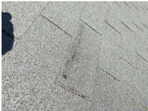
Horizontal cracking and granule loss of shingles
