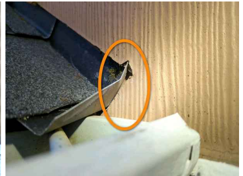
Kick out flashing is not properly sealed
