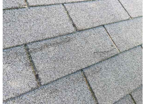
Horizontal cracking of shingles
