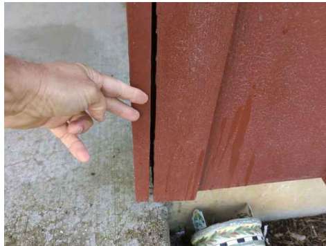
Trim is loose
