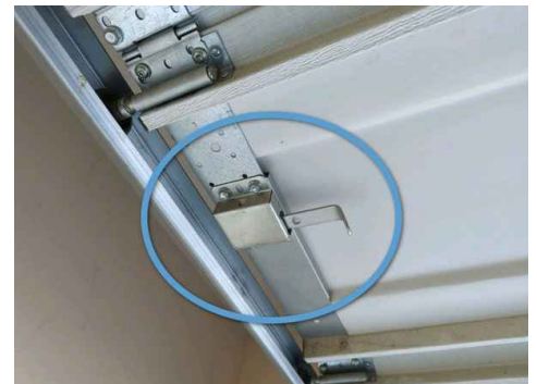
Manual lock installed on overhead door with opener
