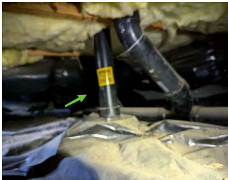
Radon piping in the crawl space
