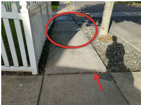
Front public walk away, tree roots have damaged sidewalk
