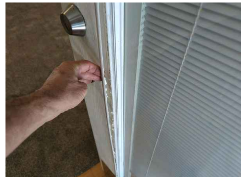
Loose trim, damaged
