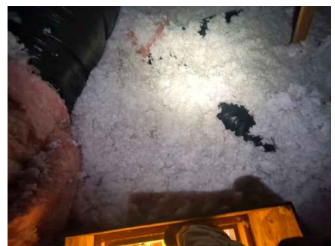
Insulation tamped down from foot traffic
