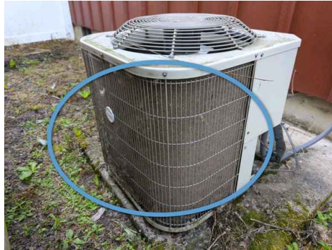
Compressor fins clogged with dust and debris
