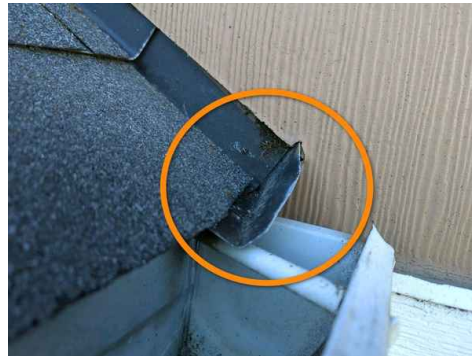
Undersized and inadequate kick out flashings
